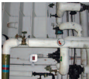
Asbestos insulation on pipes
